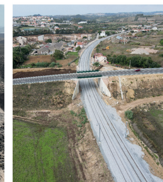
José Guilherme Modernization of the Mira-Sintra Meleças-Torres Vedras rail section of the Western Line. Portugal.
