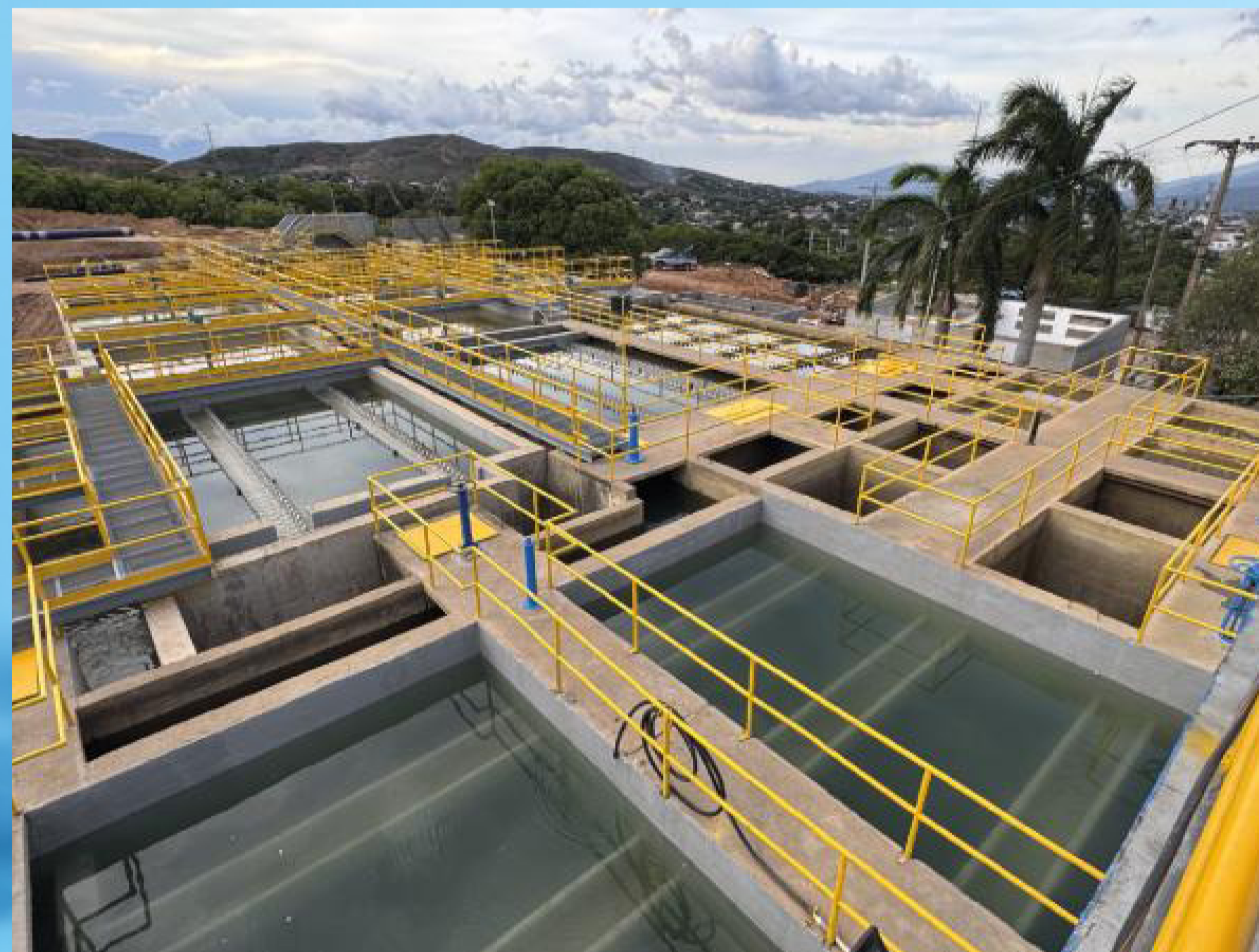
Villa del Rosario Water Treatment Plant (Colombia).
